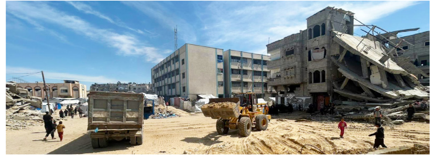
Above: Construction begins on an early years centre in Khan Younis, southern Gaza, thanks to the generous support of the El-Erian Family Foundation. Image credit: Palestinian Early Childhood Education Program (PECEP).
